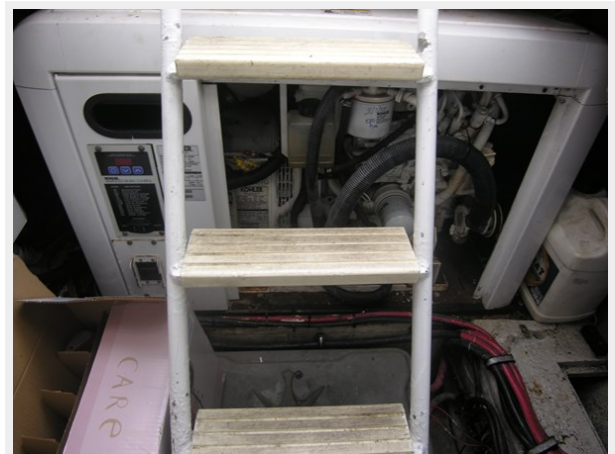
Generator Engine Room
