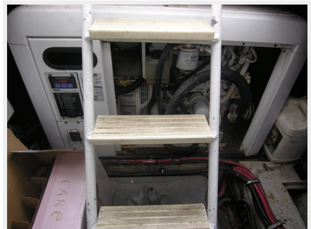
Generator Engine Room
