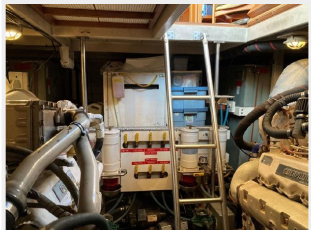
Engine room looking forward
