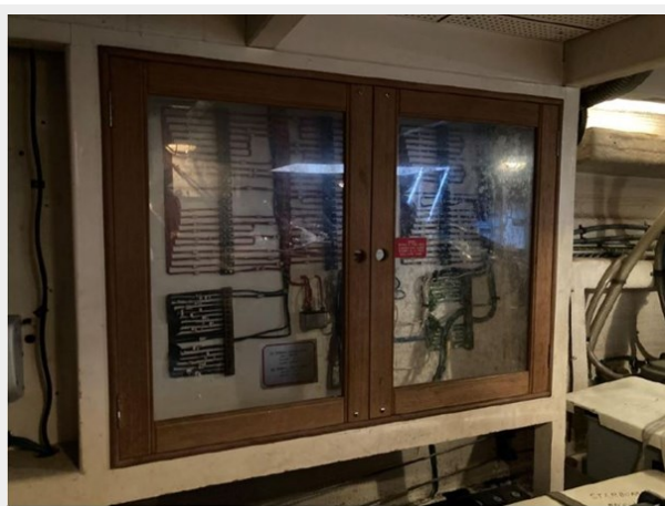
Engine room wiring (2019)
