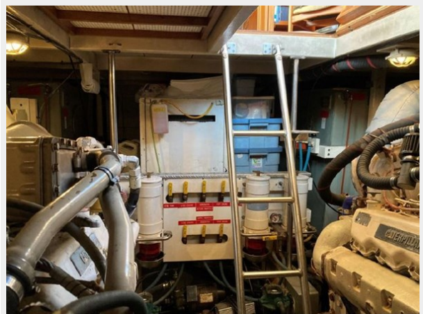
Engine room looking forward
