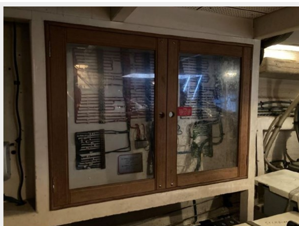
Engine room wiring (2019)
