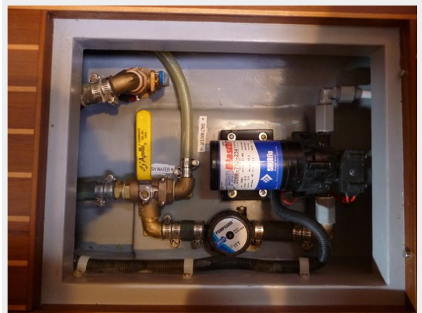
Deck washdown pump with fresh/salt water valve
