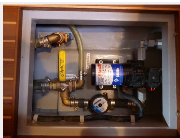
Deck washdown pump with fresh/salt water valve
