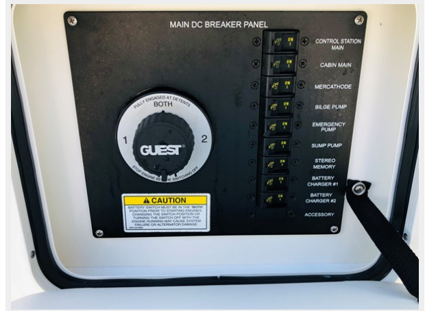
DC Breaker Panel and Battery Switch
