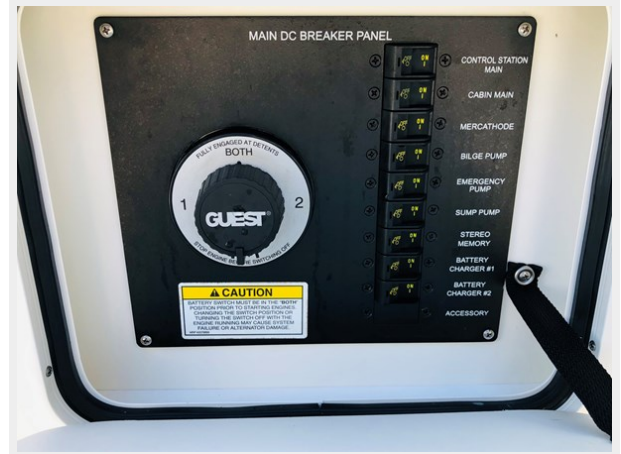
DC Breaker Panel and Battery Switch
