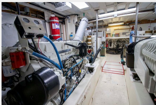
Engine Room Starboard Aft
