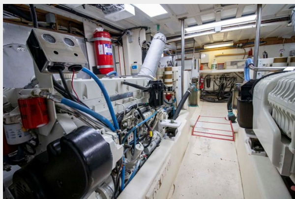
Engine Room Starboard Aft
