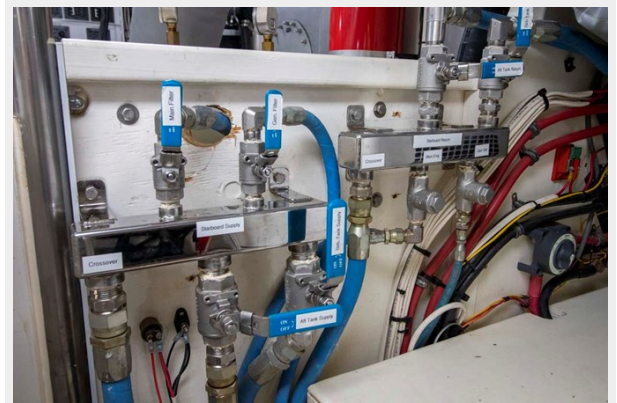
Starboard Fuel Manifold
