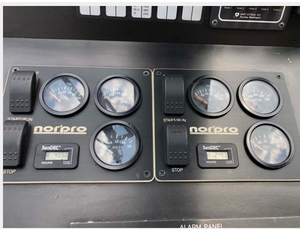
Generator Control Panel
