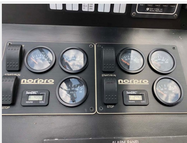
Generator Control Panel
