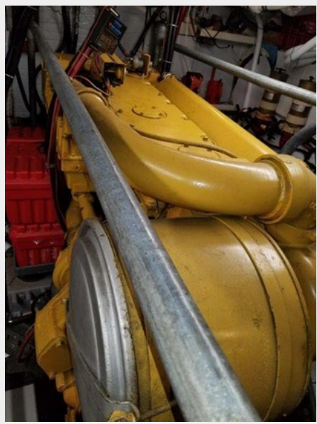
Port Side Main Engine
