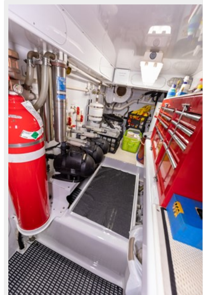
Pump Room Port
