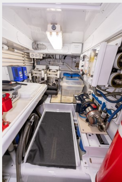
Pump Room Starboard
