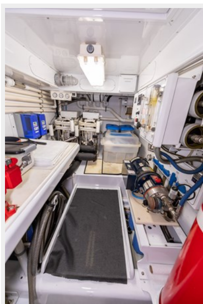
Pump Room Starboard
