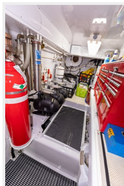
Pump Room Port
