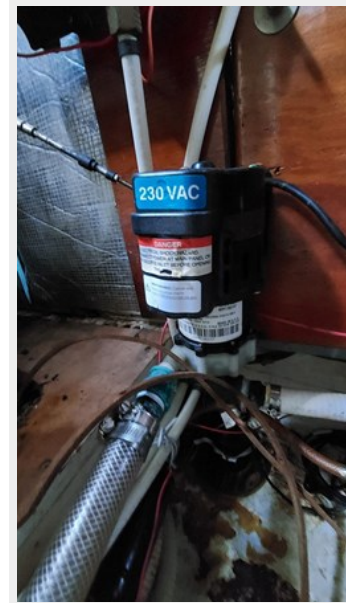
85 HVAC seawater pump
