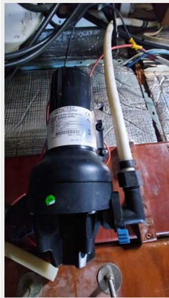
84 Fresh water pump
