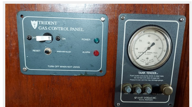
28 Tank Tender and LPG Remote Switch
