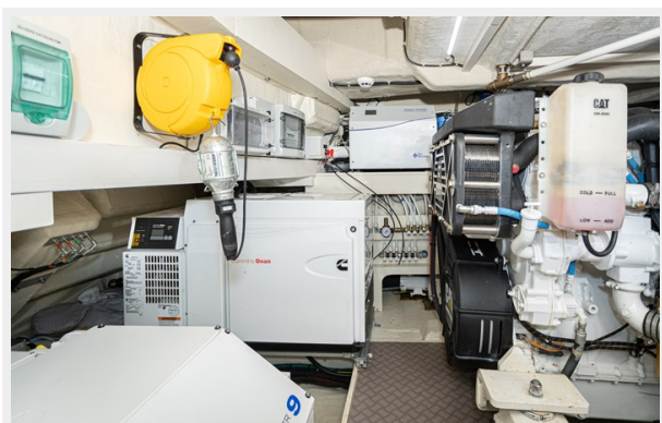
Engine Room - Generator and Watermaker
