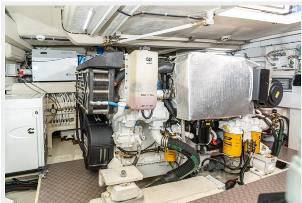
Engine Room - Port Engine
