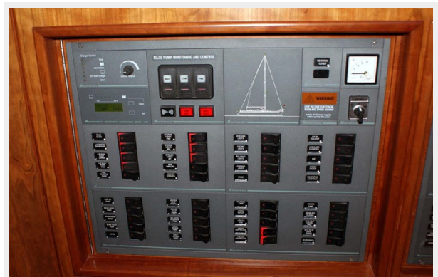
Main DC Panel
