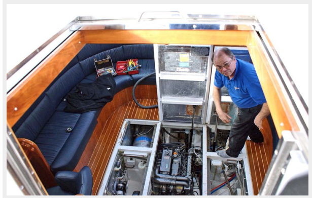
Main Salon Engine Access
