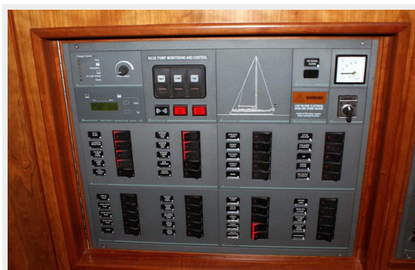
Main DC Panel
