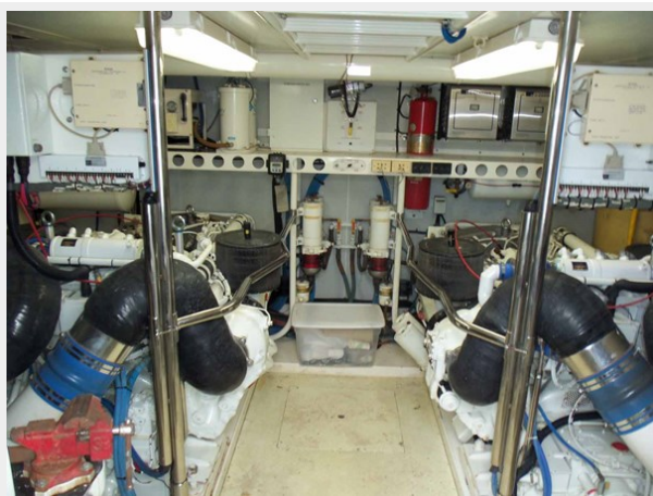
Engine Room Looking Forward
