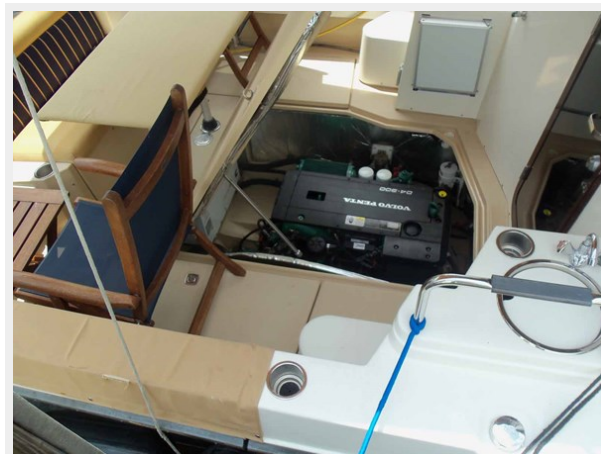
Engine Room Access
