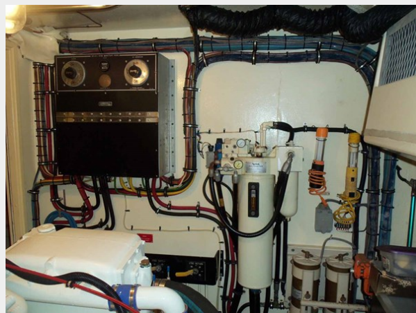
Starboard Engine Room Forward
