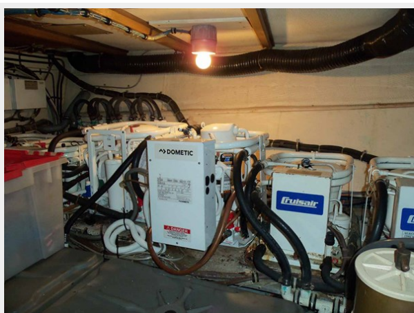
ACs in Generator Compartment
