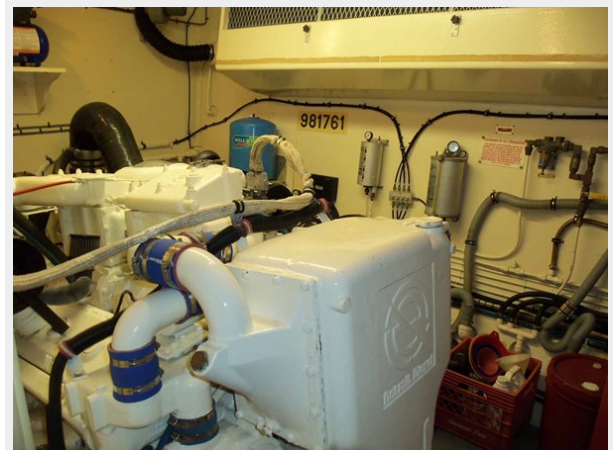
Port Engine Room
