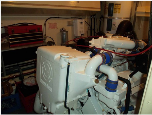
Starboard Engine Room
