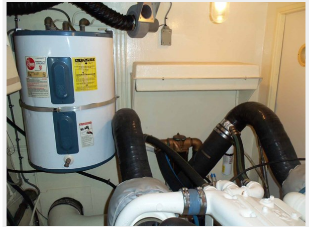
Starboard Engine Room Aft
