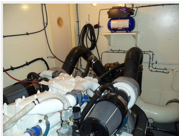
Port Engine Room Aft
