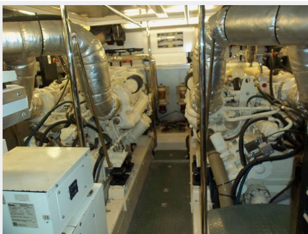
Engine Room Looking Forward
