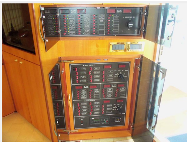
Starboard Side Electrical Panel
