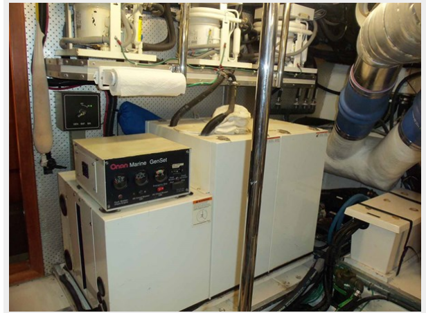
Generator Aft of Port Engine
