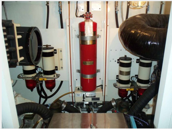
Engine Room Center
