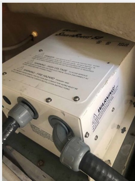
Charles Boost Transformer
