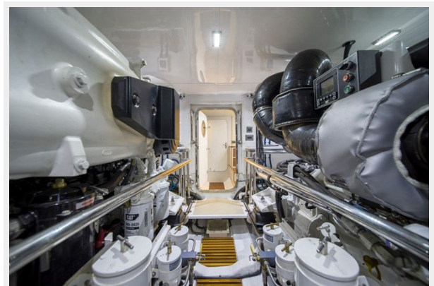
Engine Room facing Aft
