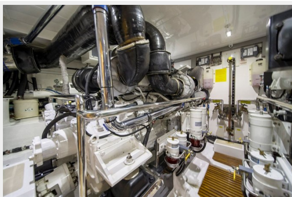
Engine Room facing Port
