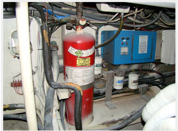
37. Port & Starboard Fire Suppression System
