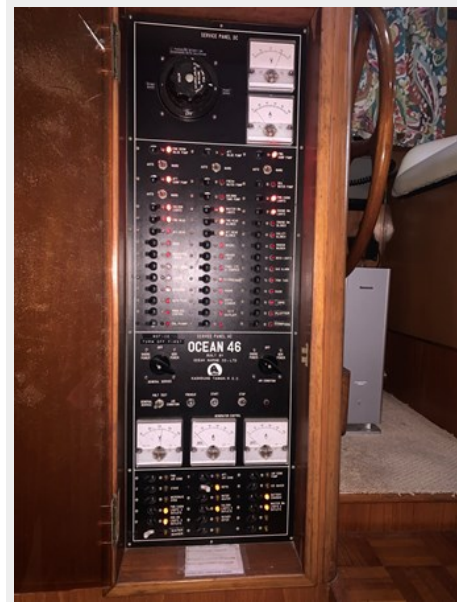
Main Electrical panel
