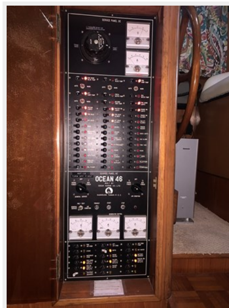
Main Electrical panel
