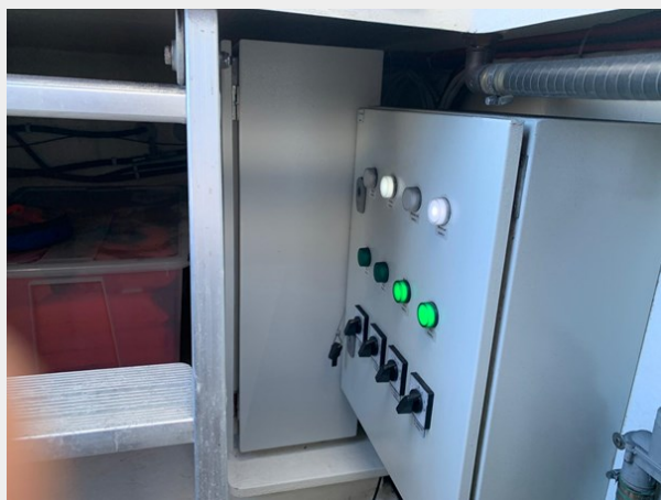
electric board engine room
