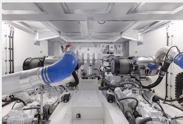
M 70 Engine Room
