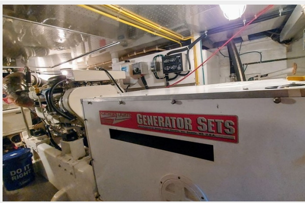
093 New Vector Engine Room Starboard
