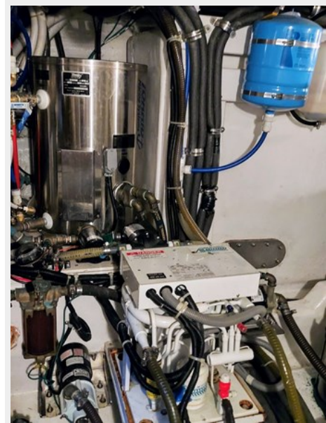
104 New Vector Waterheater and Main AC compressor
