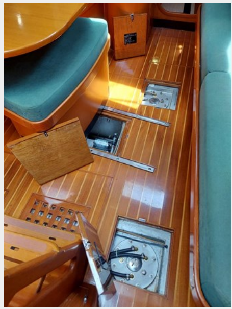
1110 Night Flight Tank and Pump access
