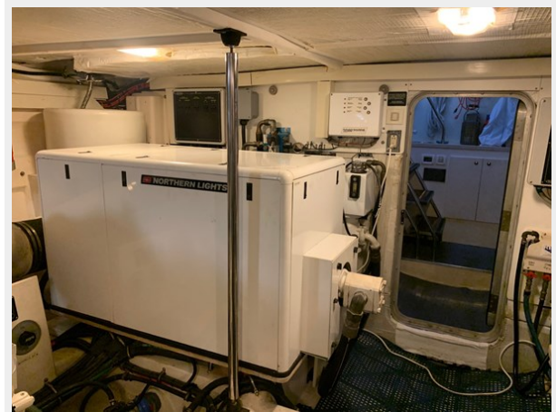
Engine Room 20 kW Generator
