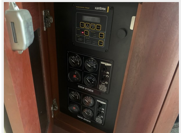
Generator Remote Start Panel
