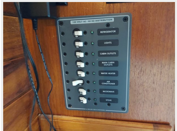
0071 switch panel (galley)
