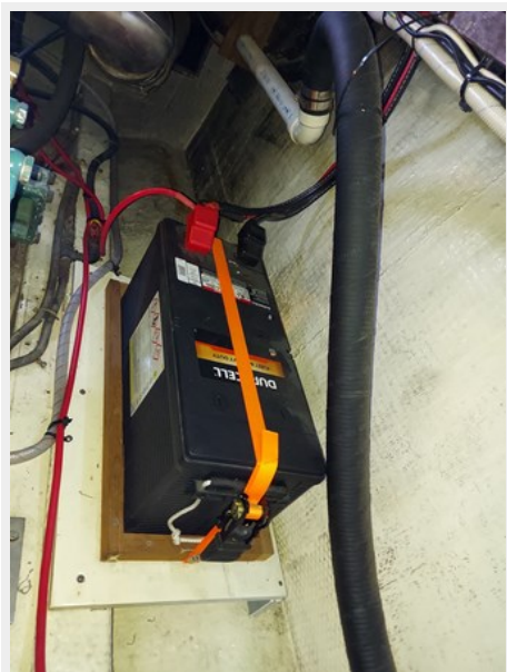
0129 Engine Room battery
