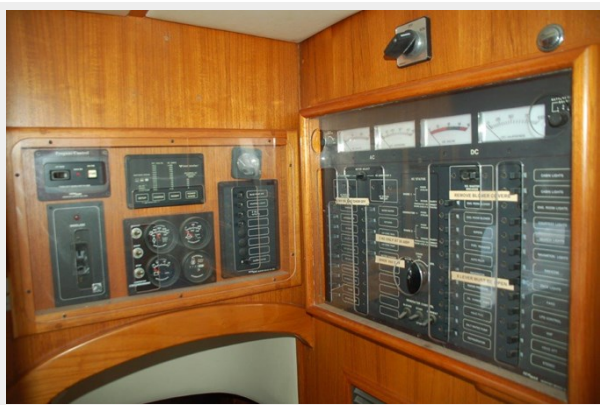
Main Electrical Panels
