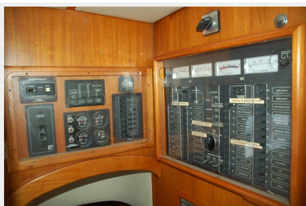
Main Electrical Panels
