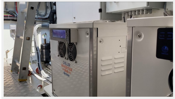
Air Conditioning chillers
