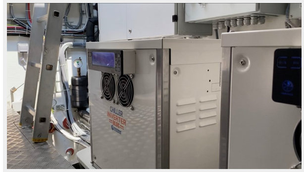
Air Conditioning chillers
