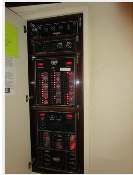
Companionway Electric Locker
