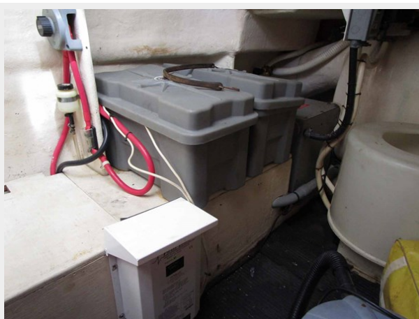
Stern Thruster Batteries
