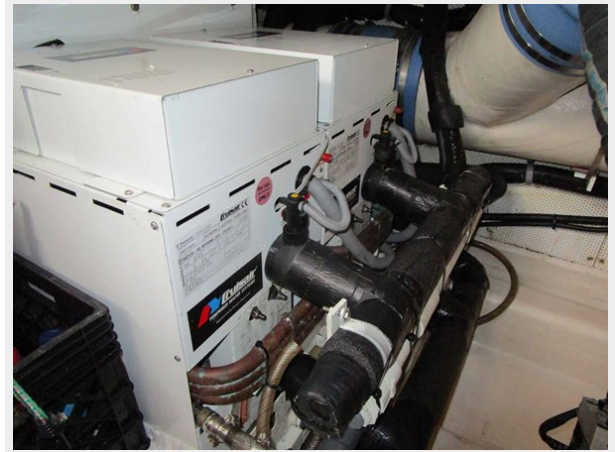
New AC Chillers
