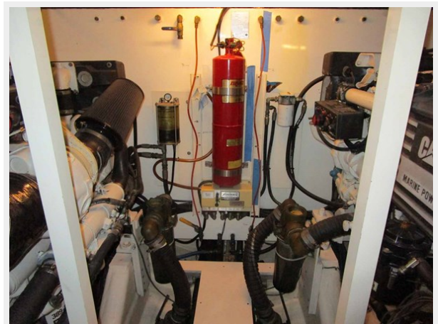
Center Engine Room
