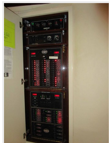
Companionway Electric Locker
