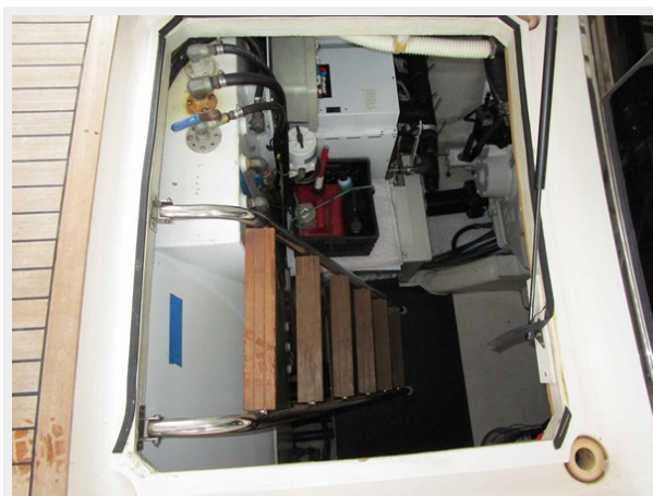
Engine Room Entrance
