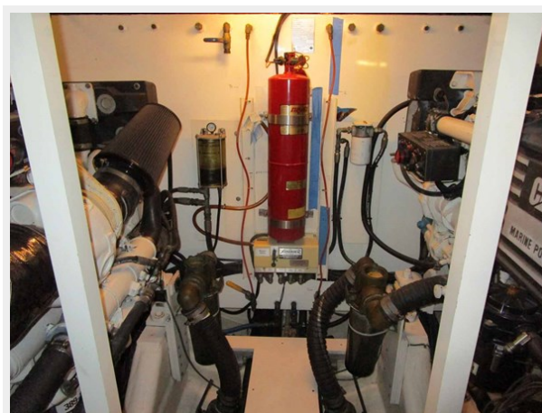
Center Engine Room
