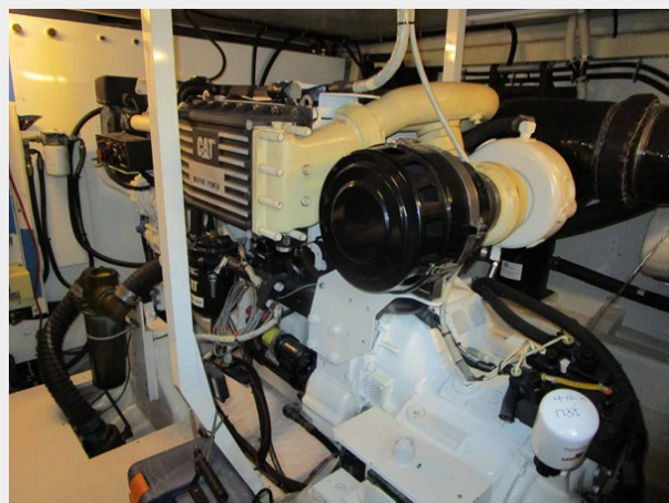
Starboard Engine Room
