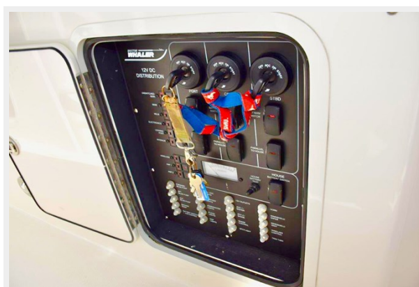
Battery panel (12v DC)
