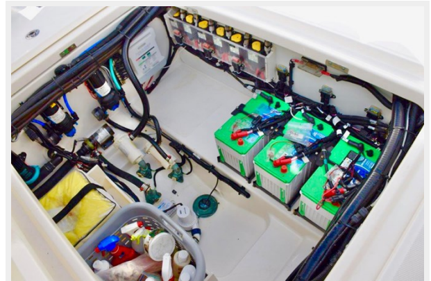
Batteries and equipment under cockpit deck
