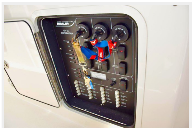
Battery panel (12v DC)
