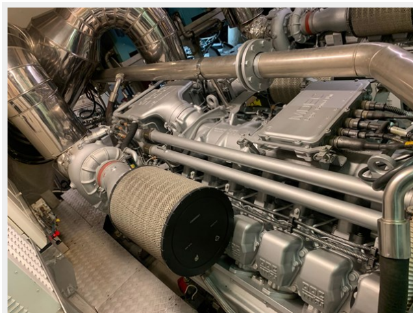
Little Zoe - Engine Room Starboard Engine
