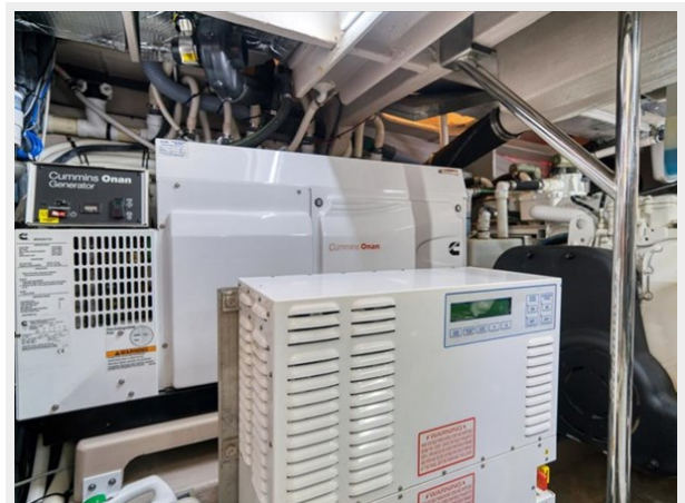
A/Sea Shore Power Converter
