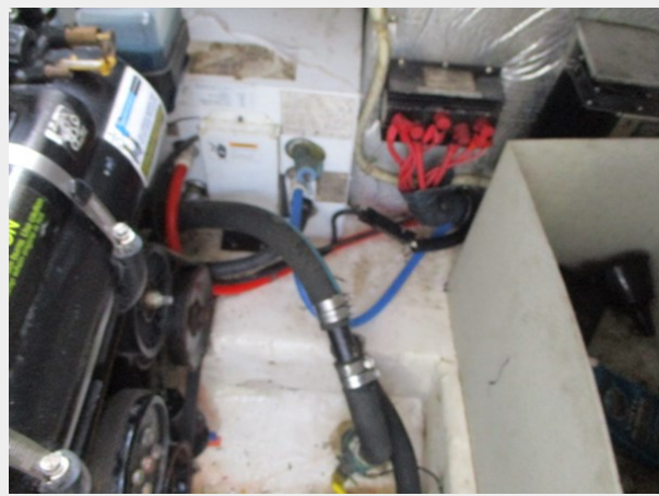
33. 30' Rinker Waterheater, Battery Charger and Bidge
