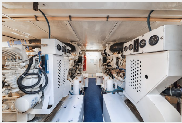
Engine Room Looking Forward
