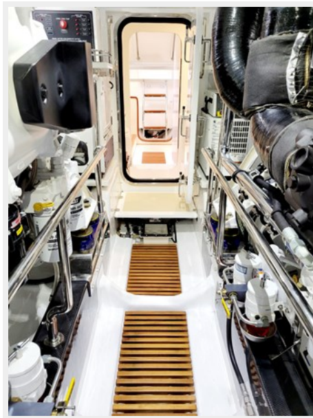
Engine room looking Aft
