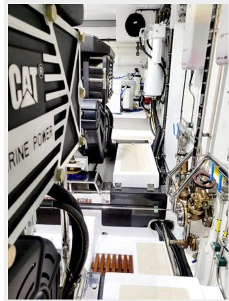
Engine room forward crossover
