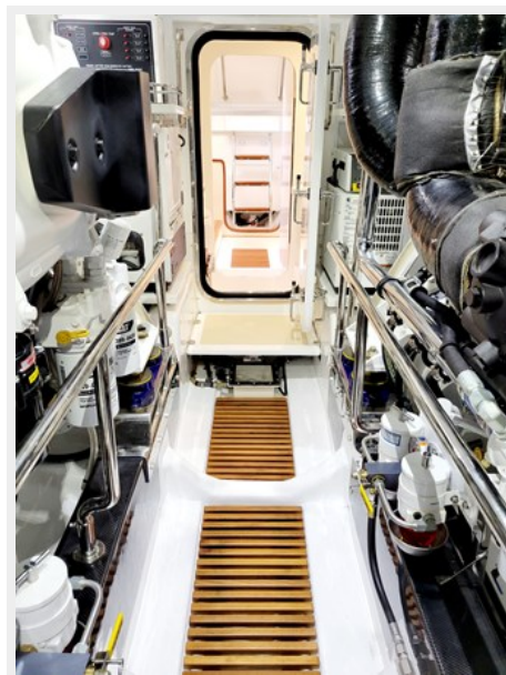
Engine room looking Aft
