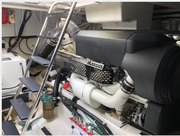
Engine Room Access
